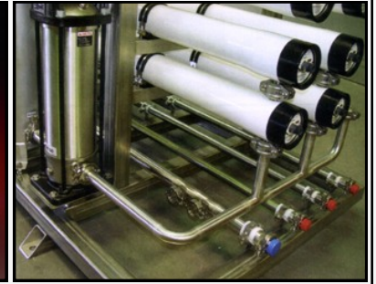
AWT skid showing orbitally welded stainless steel tubing
